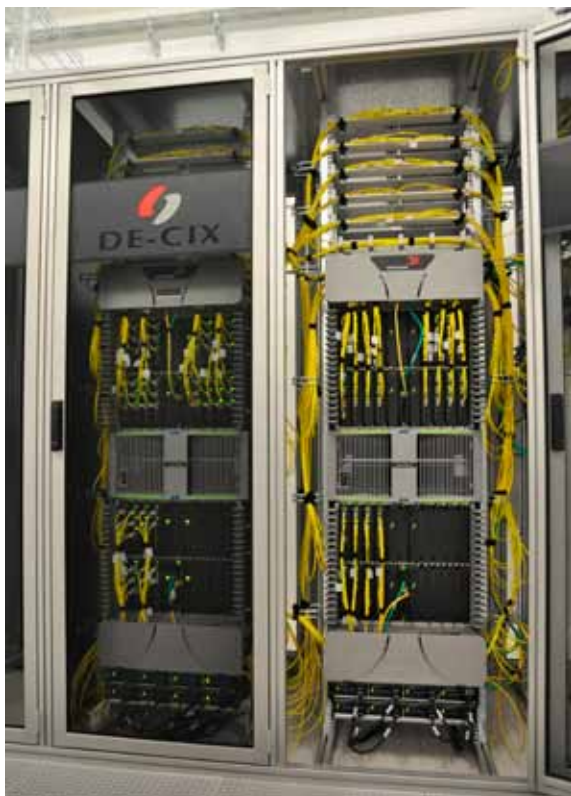
One of two core switching sites at DE-CIX. The MLX-32's provide up to 512 line rate 10GE ports
